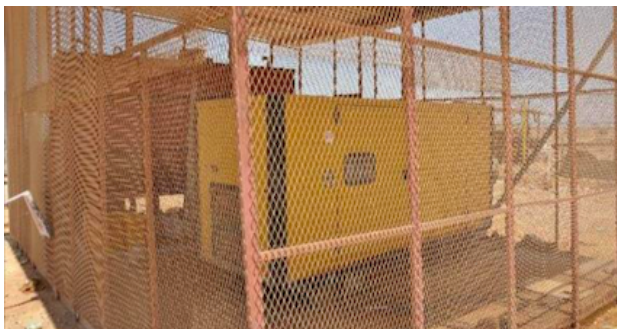
Figure 1: A generator in Markazi settlement, Djibouti.
